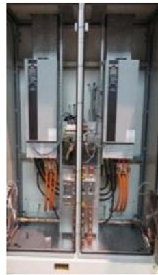
Frequency converters compressor drives + main power connection
