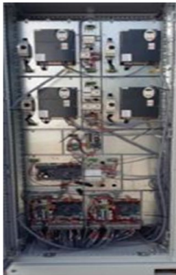
Frequency converters fan drives + Pump drives + electronic boards
